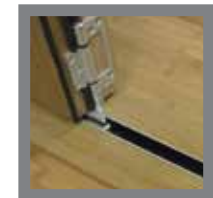
Your flooring butts up neatly to the oak sill, which has a special aluminium sub-sill for easy fitting and extra strength
